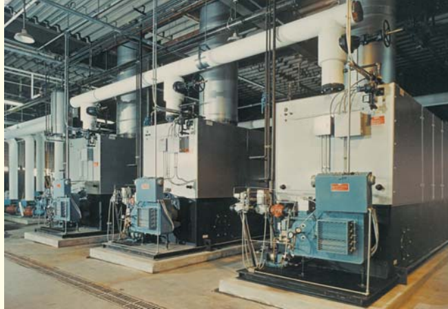
Three Bryan Boilers provide 56,250 MBH to heat 495,000 sq. ft. expansion of Milwaukee's General Mitchell Field air terminal.
